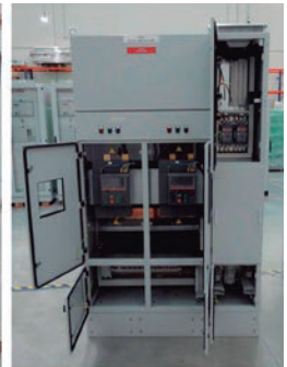
Battery Connection Panel
